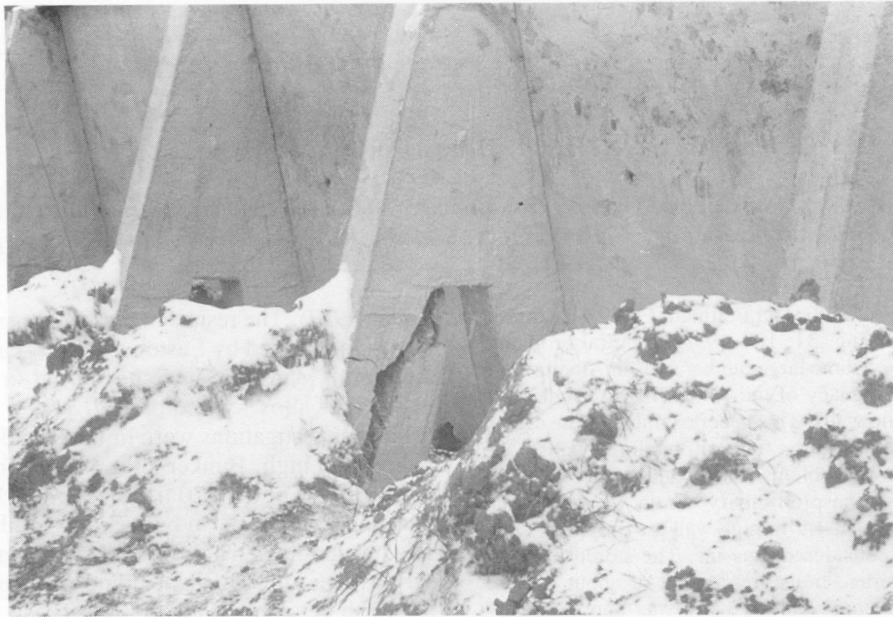
Figure 1. Break in the top of the rear leg of a bunker silo support frame; crack initiated by a combination of high negative moment and shear.
