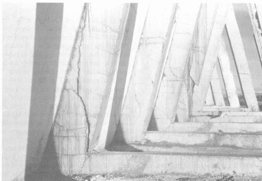
Figure 4. Cracks in the bottom of the front leg of a bunker silo support frame; cracks initiated by a combination of high negative moment and shear.
