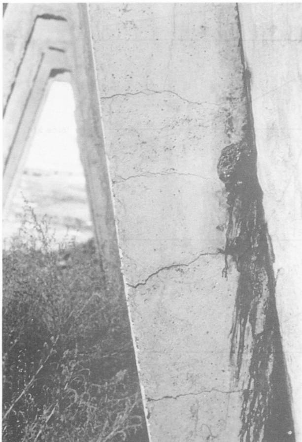
Figure 3. Positive moment cracks in the front leg of a bunker silo support frame.
